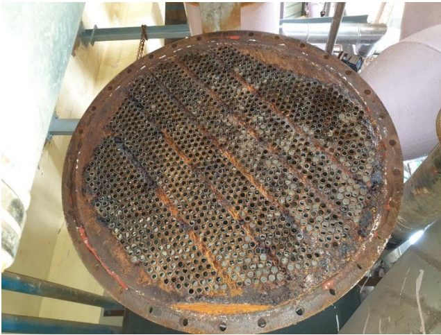
Tube sheet suffering from corrosion and chemical attack
